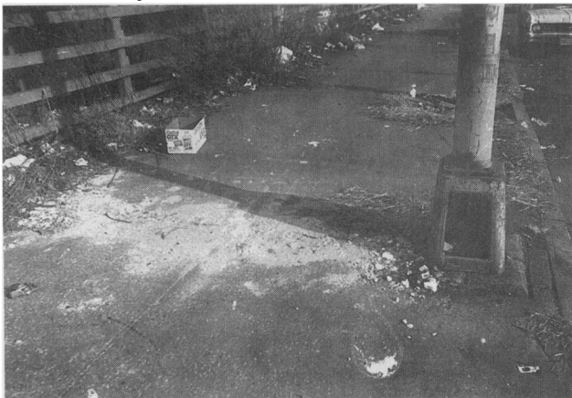
5. A lamppost that has been opened to connect electricity to a makeshift shelter; sand is used to hide the wire.
